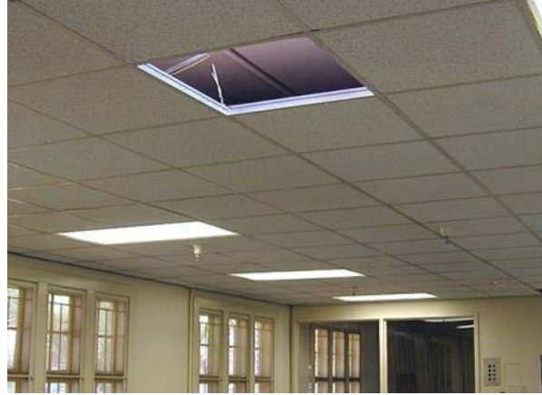
Lay-in ceiling tile
