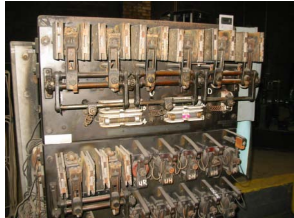
Transite Blocks in Elevator Switchgear
