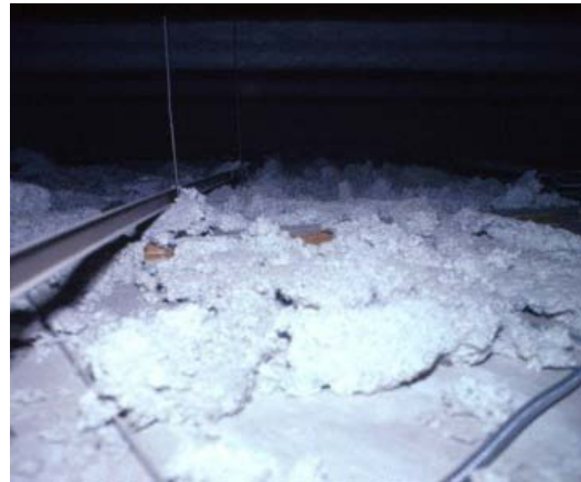
Debris from fireproofing on top of ceiling
