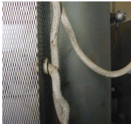
High Voltage cable insulation
