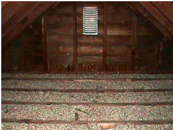
Vermiculite attic insulation
